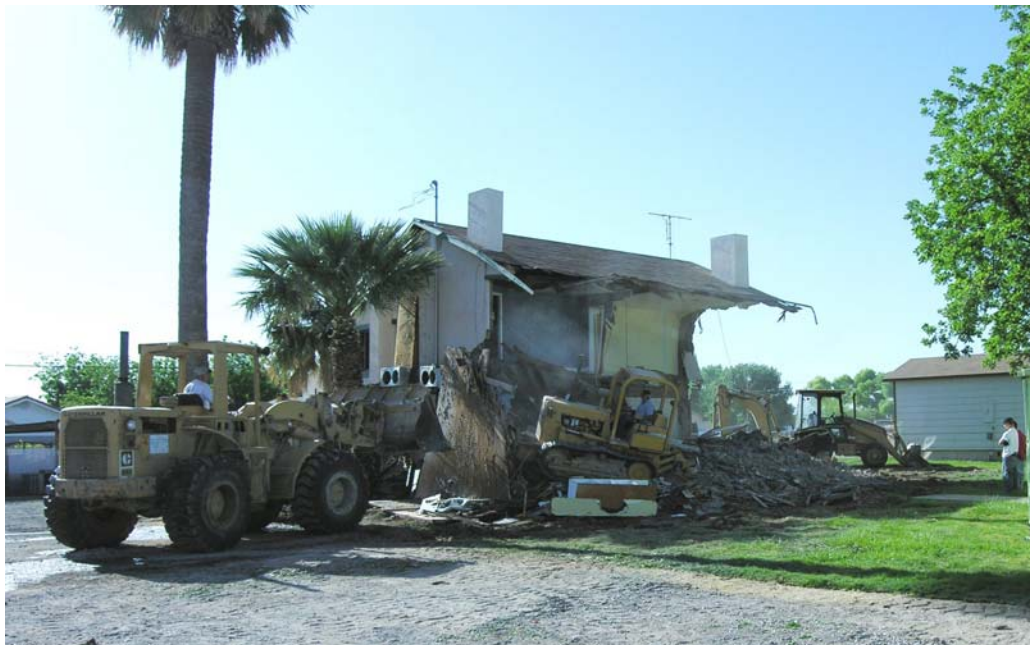
April 29, 2006, The Brigham Whitmore house was demolished just two days before Archaeology Awareness and Historic Preservation Month.
